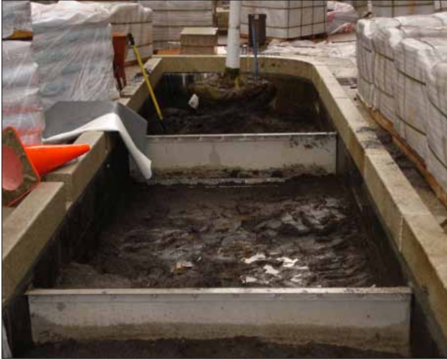
Foot traffic during construction can easily compact soils, especially clay, reducing or eliminating infiltration capacity.
